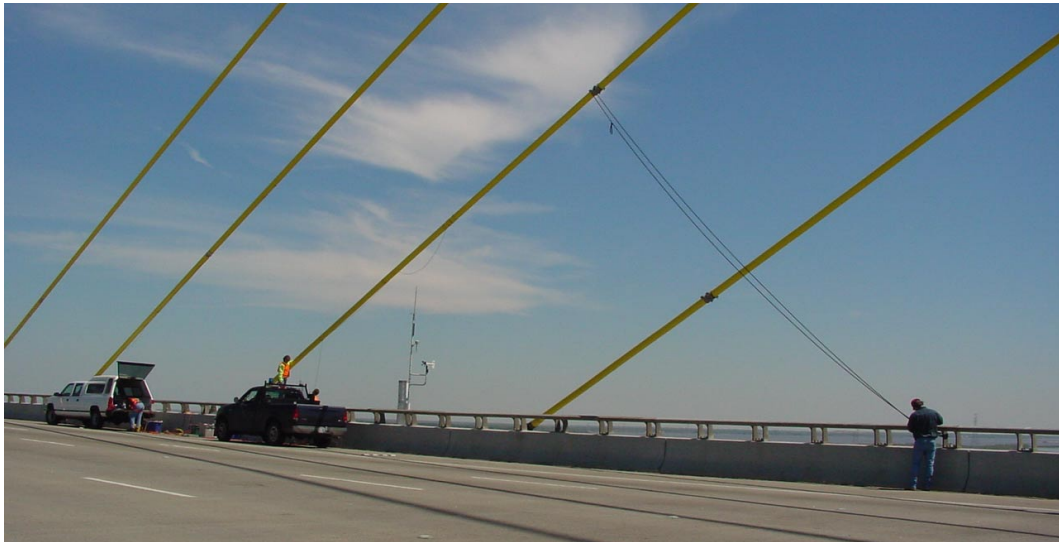
Figure 4.16: Pluck Test of Cable A22S
