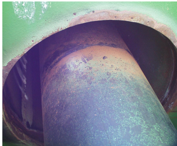
Figure 3.13: Indentation in Polyethylene Sheath at Anchorage Box
