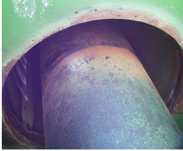
Figure 5.9: Example of Indentation in Polyethylene Sheath at Anchorage Box Opening
